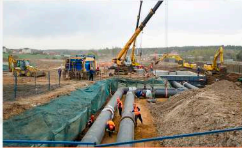
WATER MAIN ALONG THE KALUZHSKOYE HIGHWAY
